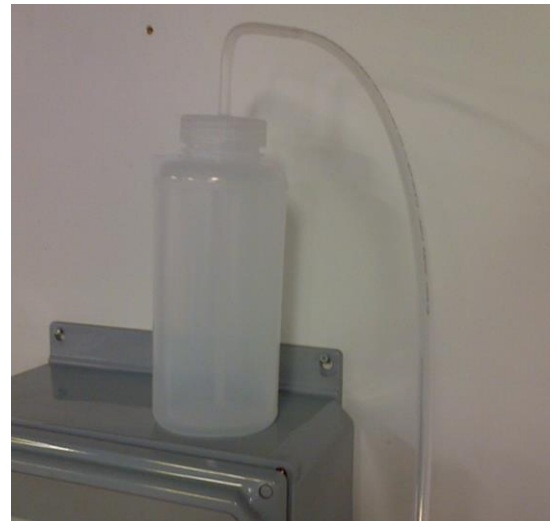
Figure 14.6: Bottle on top of cabinet
